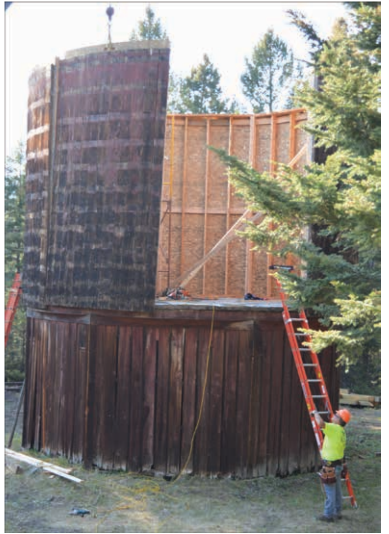
Right, Cody moves a ladder into place to advance on the restoration work. Clearly visible on the outside of the tank are lighter bands of color where metal bands had been in place. Those were painstakingly removed earlier this summer as part of the effort to stabilize the old tower to save it for future generations to appreciate. (Photos by Bruce Bell and Dr. John Smith)
